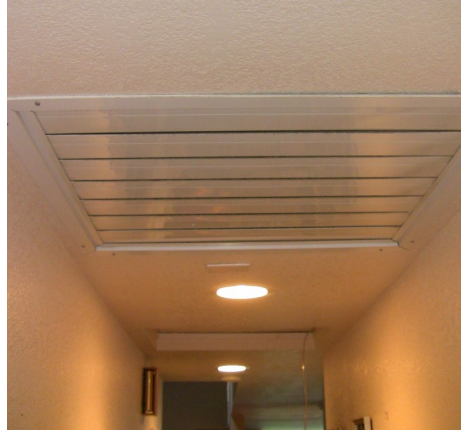
Figure 4-38: Whole-House Fan With Barometric Damper
