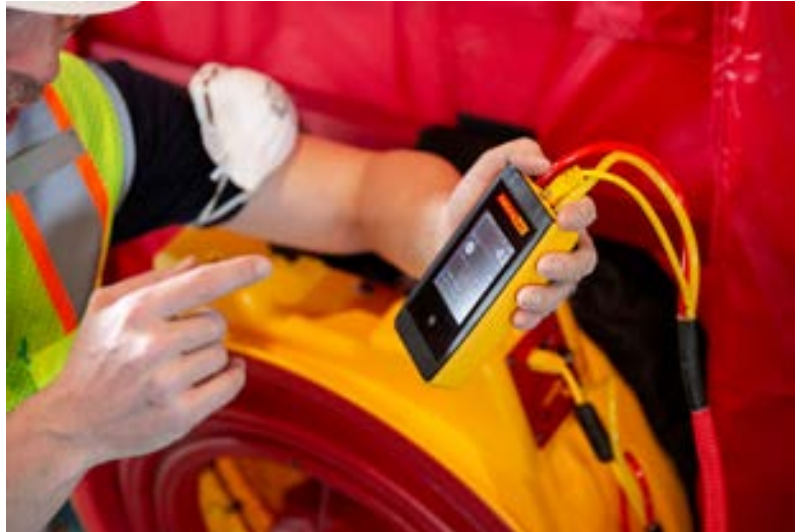
HERS Verified Blower Door Test – Envelope leakage, when modeled, must be verified by a third party HERS rater. Source: California Energy Commission
