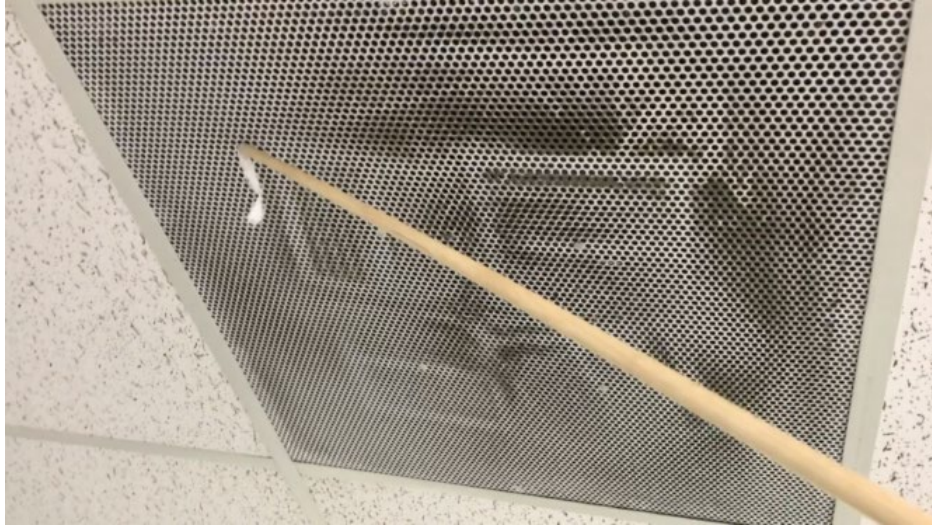
Figure 5. Checking that air is entering the room from a ceiling supply air diffuser with an airflow indicator.
