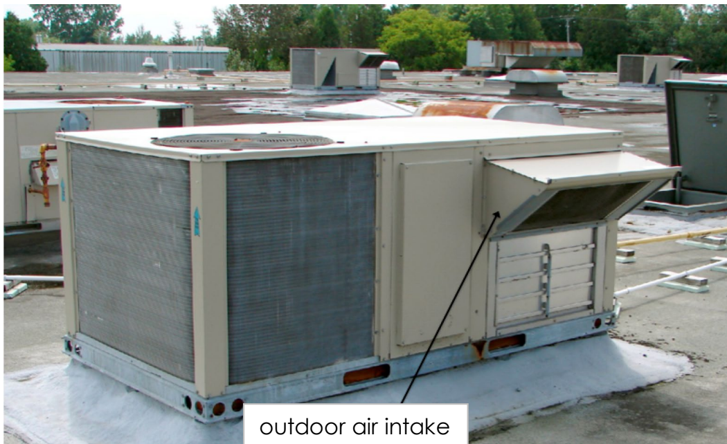
Figure 4. Outdoor air inlet for a typical rooftop HVAC system.
