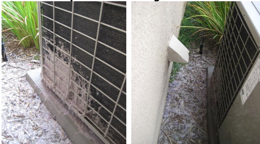
Figure 4-2: Noncompliant Condensing Unit Clearance from Dryer Vents
