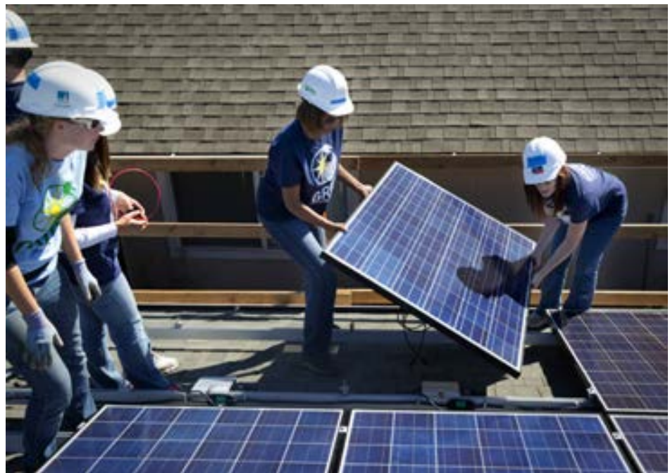
Solar Panels Installed on a Low-Rise Residential Building – Solar photovoltaic systems are prescriptively required for all newly constructed low-rise residential buildings under the 2019 Energy Code.
