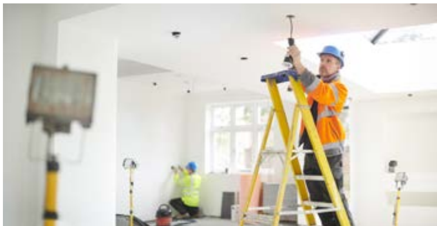
Lighting Alterations – Requirements for these alterations have been modified for simplicity.
