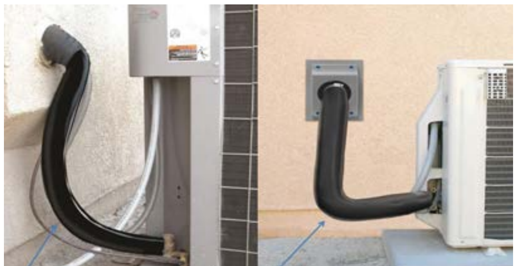
Pipe Insulation Protection – Insulation must be protected from damage due to sunlight, moisture, equipment maintenance, and wind, according to Section 120.3(b) of the Energy Code.
