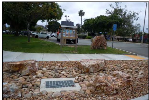
Infiltration basin installed as part of the "A" Avenue Green Street and Pedestrian Pathway Project
