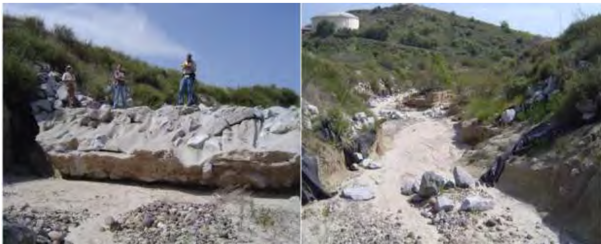
Figure 3-2. Undermining of grade control and erosion of banks downstream of structures intended to stabilize a particular stream reach. Left photo is looking upstream at drop structure; right photo is looking downstream from the drop structure.
