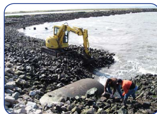
The City has conducted a series of engineering studies to determine the best ways to protect neighborhoods during big storms and sea level rise.
